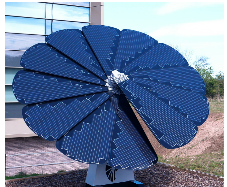
Fig. 24 - Existing solar panels installed on SEZ site.
