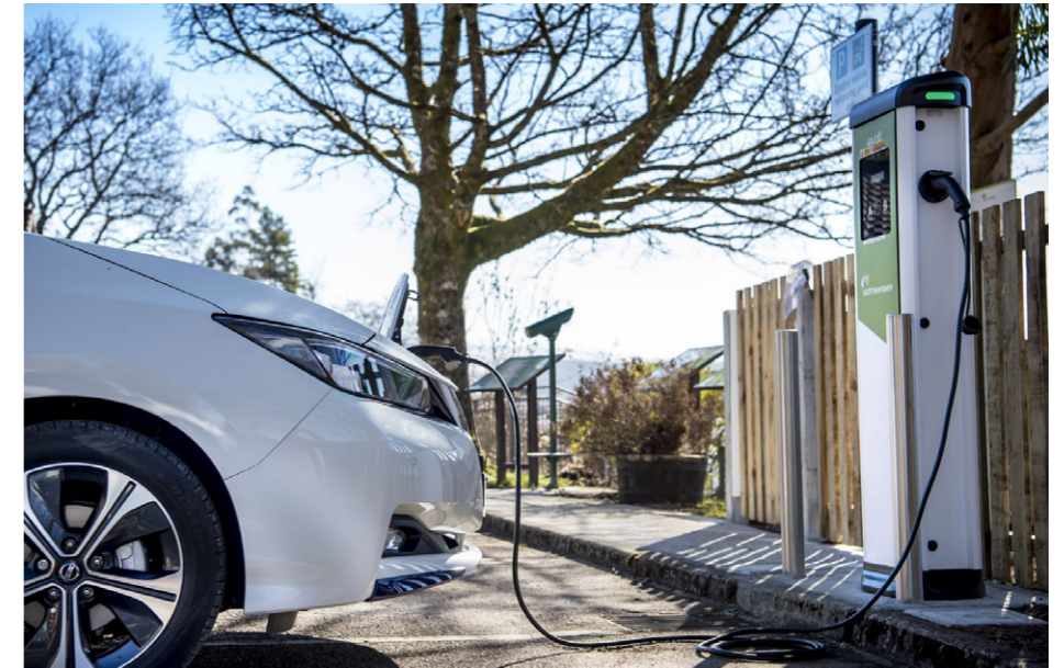
Fig. 22 - Electric vehicle charging point.
